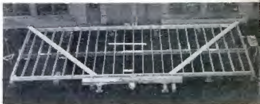
In structures of average size, two diagonal braces have been found to be ample floor bracing for conventional floor framing. Larger buildings and those with long floors require more
